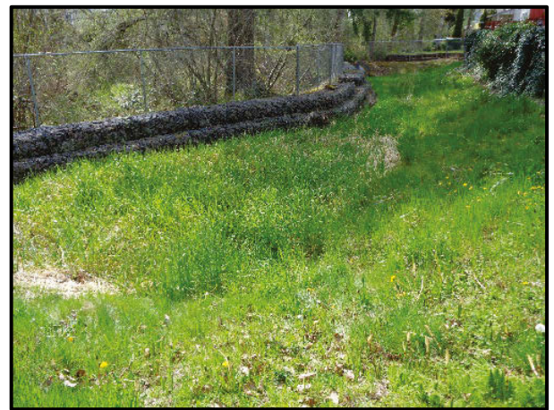
Before: Facility is overgrown and filled with heavy sediment.
