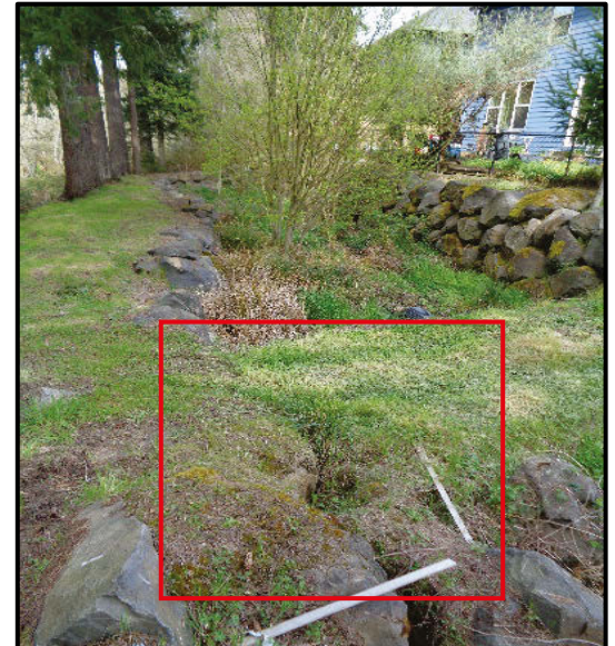
Before: red box indicates the depression in the ground.
