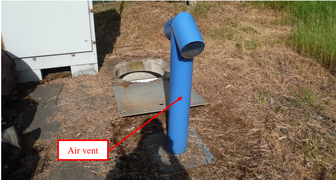
Figure 8.10 – 1st Avenue PRV Vault - Air Vent Pipe
